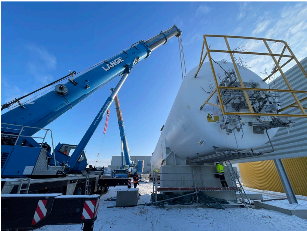
Two heavy-duty cranes have brought the 130-tonne tank into position (Photo: EnviTec Biogas AG)
